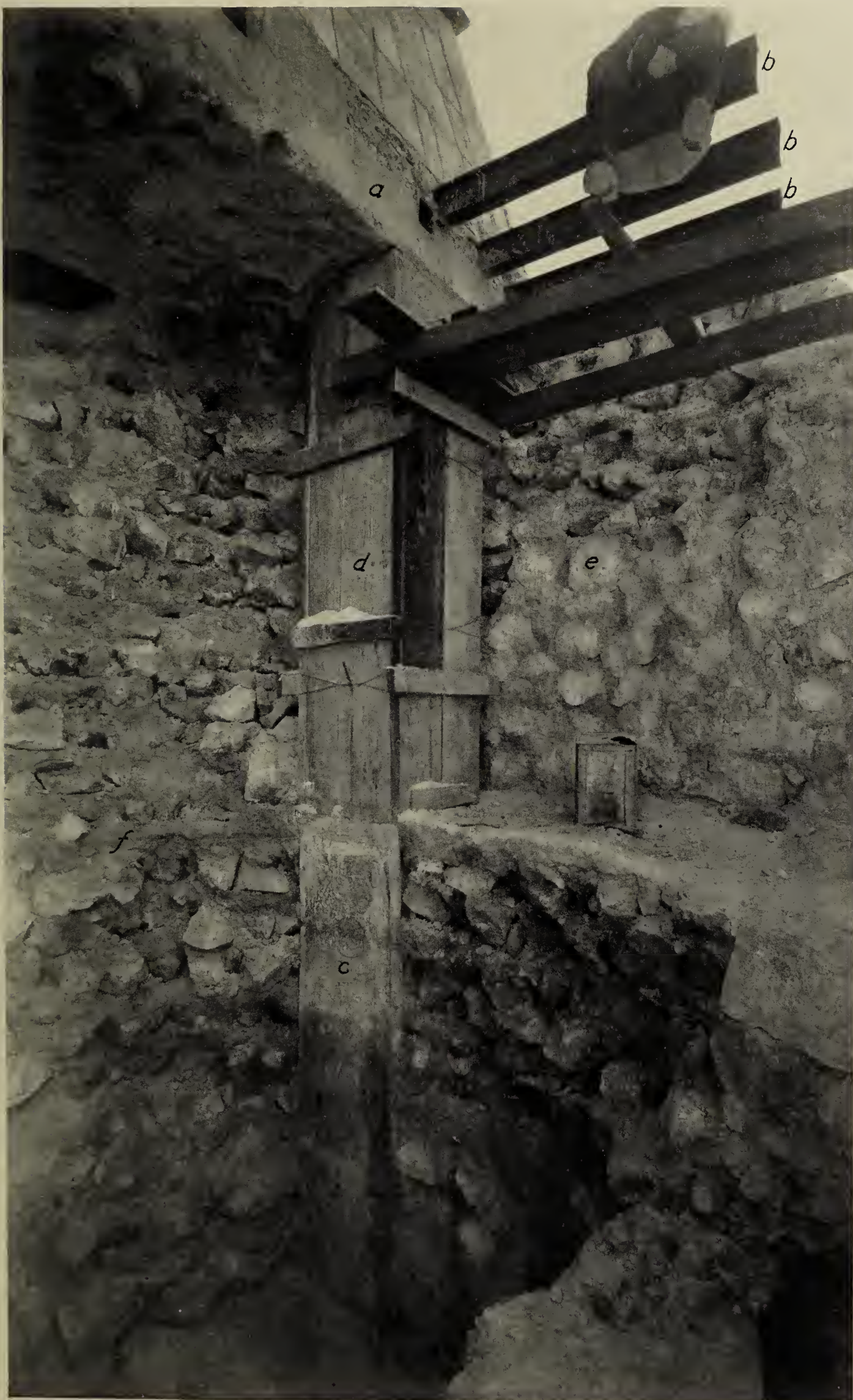
CONCRETE COLUMN CAST ON TOP OF COLUMN 5, TEMPLE OF THE CHAC MOOL
